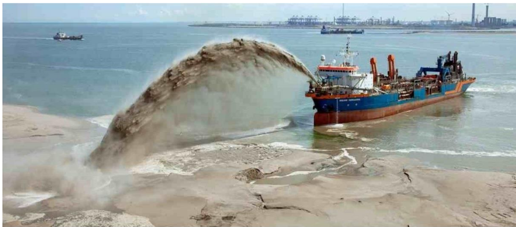
Dredging/cleaning of the sea floor and supply of sand/gravel to fill the cylinder barrier (Van Oord Ship)
